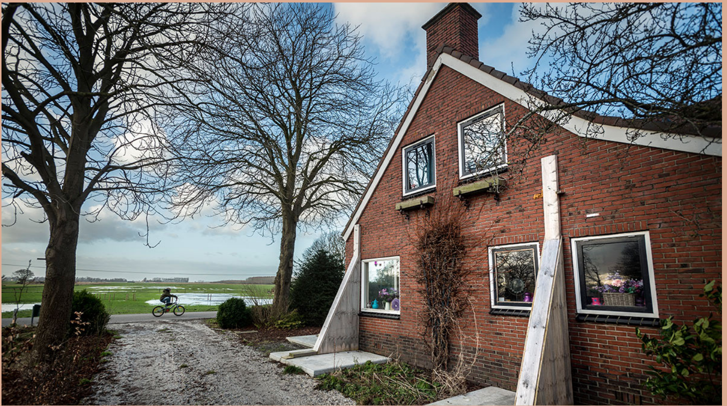
Earthquake damage to Groningen house
